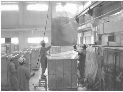
Fig.17 Containment the Radioactive Waste
