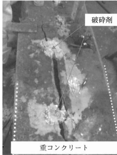
Photo 6 Destruction Process of Heavy Concrete
