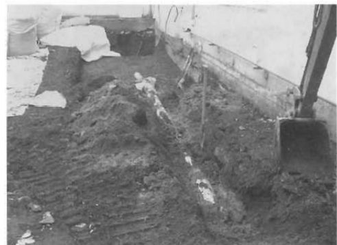
Fig.21 Removal of Pipe Under Ground, as Much as Possible Before Dismantle of Buildings
